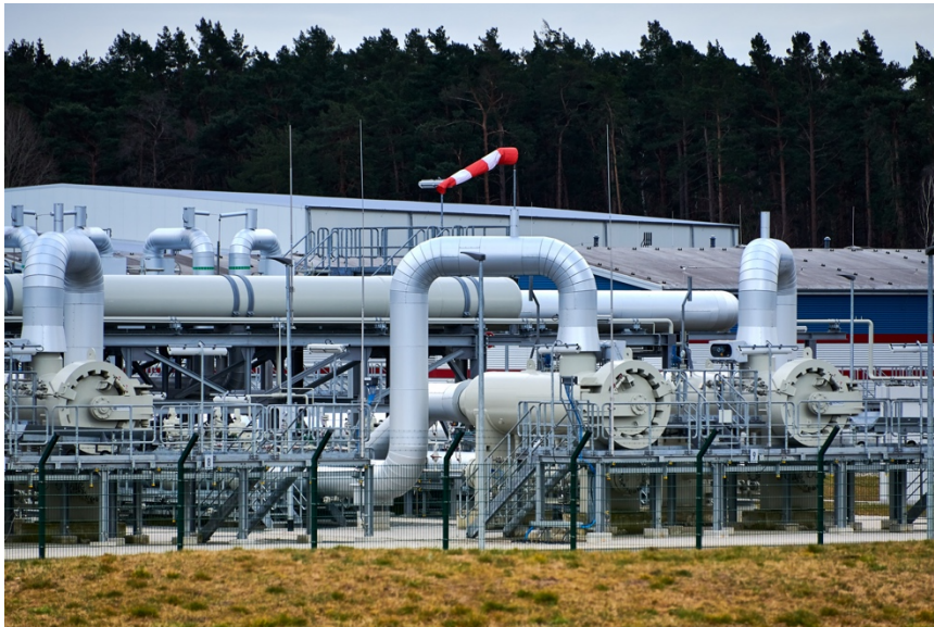
Figure 16: Lubmin, Mecklenburg-West Pomerania, Germany. Gas pipes, connections, equipment and pressure reducers at the site of Gazprom's Nord Stream 2 Pipeline landing in Germany.
